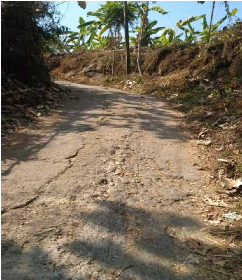
The broken road uphill.
