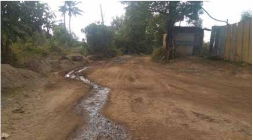
The road used by the quarry vehicles seems to be in a state of extreme disrepair.
